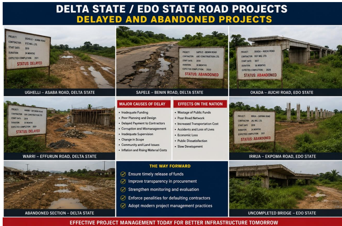
Figure 2. Primary causes of project delays in Nigerian Public Infrastructure Projects
