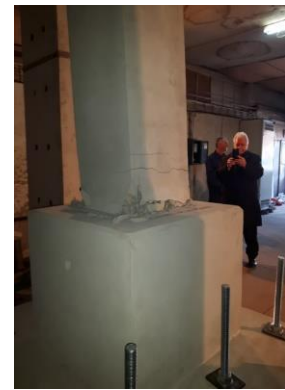
Figure 20. Heavy damage at RC column
